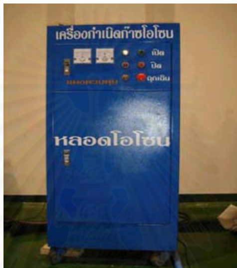
Figure 5.8 Walailuck University ozone generator
