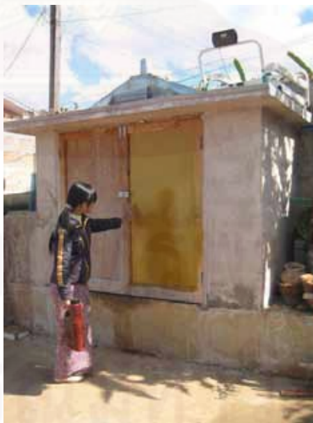
Figure 13: The Samphinong's gasoline generator room for household, and media operation use
