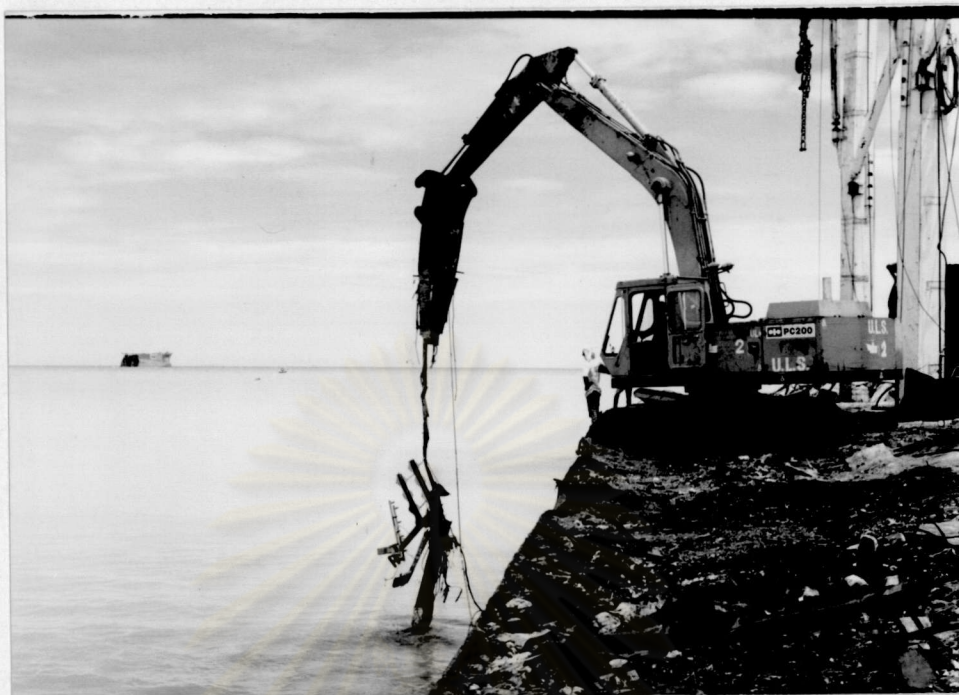
Pieces of steel directly falls into the sea and weathering.
