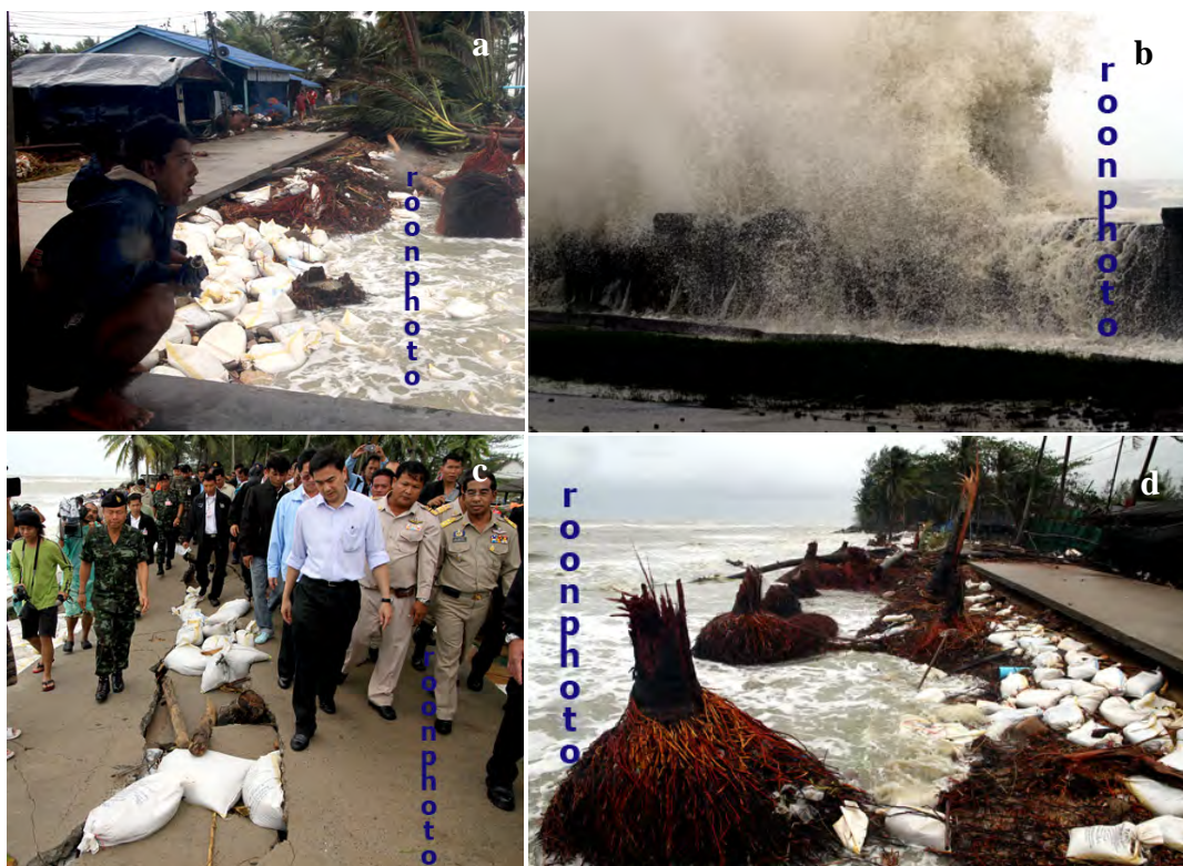
Figure 2.17 Damage from storm surge at Laem Talumphuk, Nakhon Si Thammarat province on 29 and 30 March 2011. a) A man was frightened to see the strong wave which going to destroy his house. b) Wave high 4-5 m attacked the seawall. c) Prime minister Abhisit Vejjajiva is investigating the damage at the LT village. d) Root of coconut trees were exposed due to the erosion of beach sand. (pictures from http://www.oknation.net/blog/singslatan )
