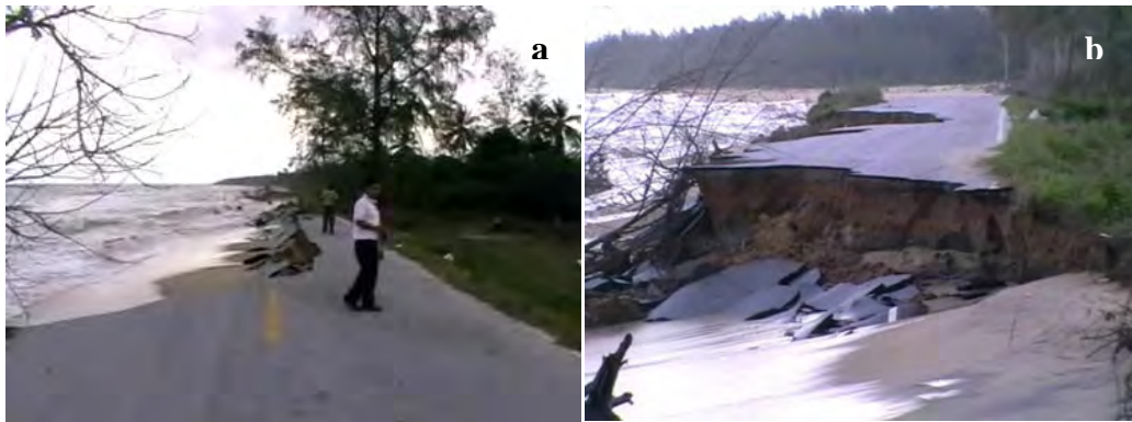
Figure 2.18 Picture a) and b) showing the destroyed road along the shoreline at Yaring district, Pattani province by strong wave from storm surge on 1 April 2011.
