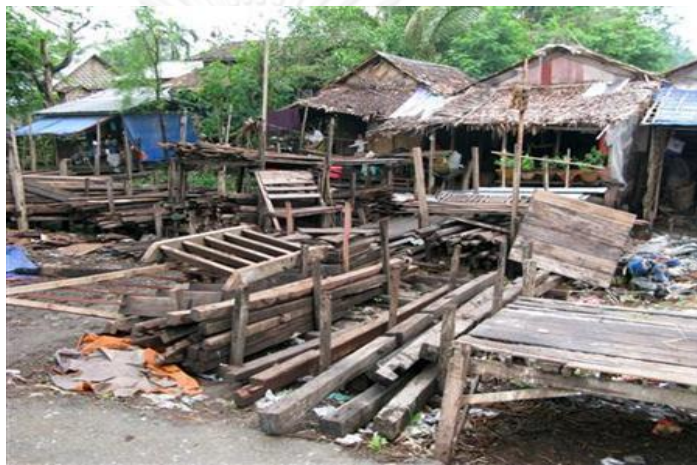
Figure 2: Cyclone Nargis damaged thousands of homes and basic infrastructure.
