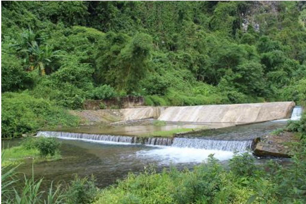
Figure 4.4 Concrete weir in Pha Tang Village, Vang Vieng district as of 6 th June 2014
