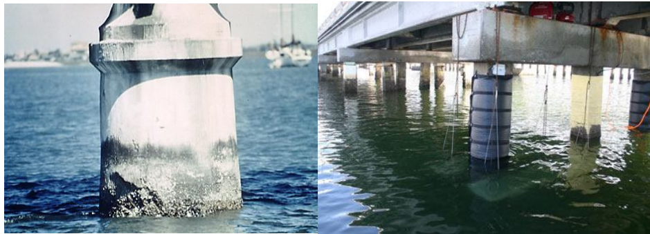
Figure 1.1: Degradation of reinforced concrete structure in marine environment
