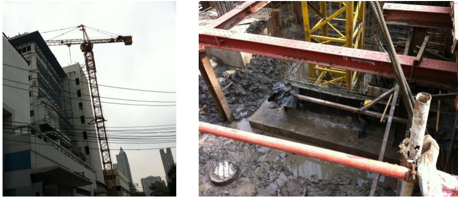
Figure 4.2 Different locations of the tower cranes: attached to the building and located in the lift core
