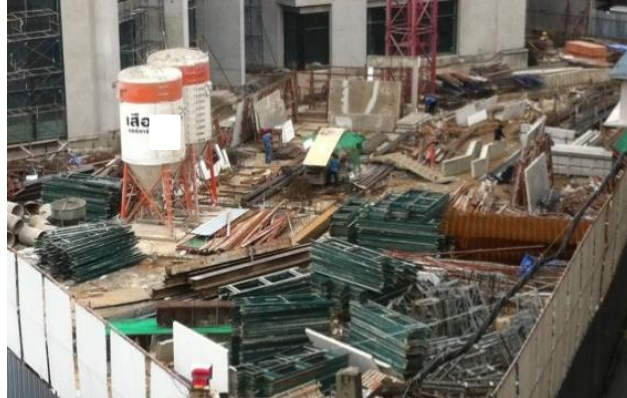
Figure 4.11 Untidy laydown area on the job site
