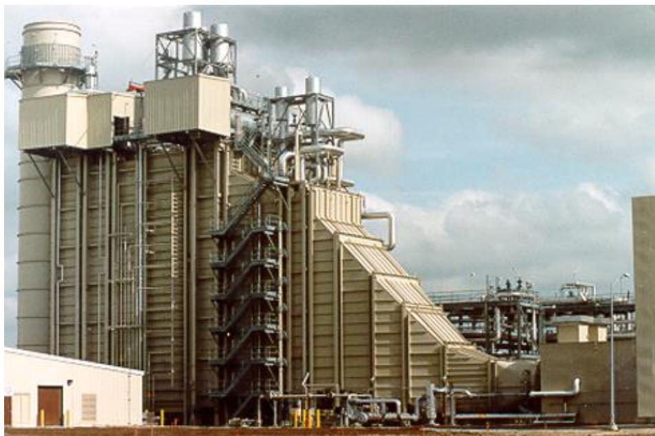
Figure 1: Heat Recovery Steam Generator
