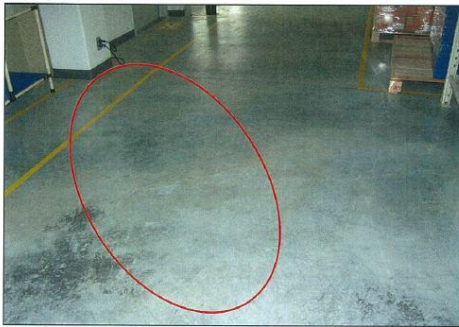
Location of floor crack at column line G/6 . ( point 1 )
