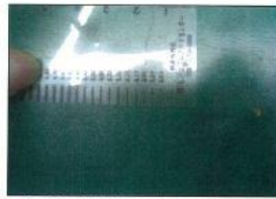
1. Crack 0.08 mm. (L=2,000 mm.)
