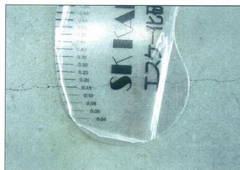
Floor crack 0.15mm long 1,750mm.
