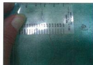
7. Crack 0.2 mm. (L=4,000 mm.)
