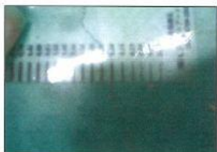
6. Crack 0.2 mm. (L=6,500 mm.)
