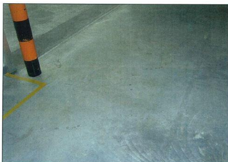
Floor crack at guard pole line G/6 . ( point 3 )
