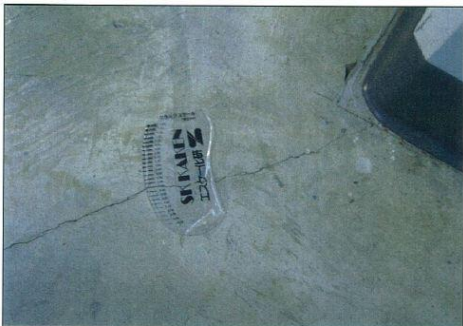
Floor crack at column line G/6 . ( point 1 )
