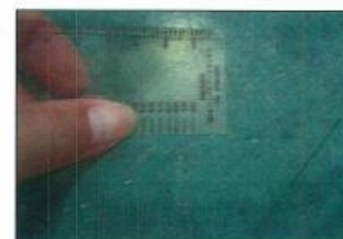
11. Crack 0.04 mm. (L=9,000 mm.)
