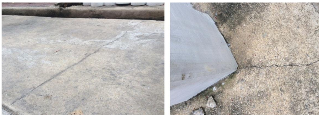
Figure 2.4: Transverse crack and re-entrant corner crack due to drying shrinkage
