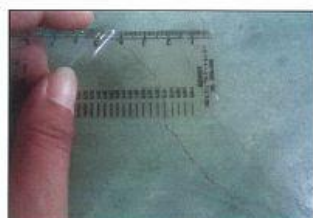
12. Crack 0.15 mm. (L=8,000 mm.)
