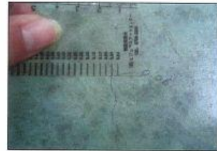
2. Crack 0.06 mm. (L=1,500 mm.)
