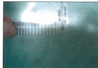
4. Crack 0.06 mm. (L=1,500 mm.)
