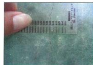
9. Crack 0.2 mm. (L=8,500 mm.)
