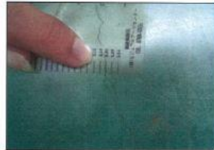
3. Crack 0.08 mm. (L=1,500 mm.)
