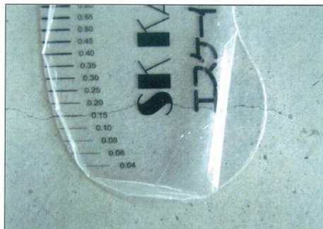
Floor crack 0.15mm long 1,640mm.
