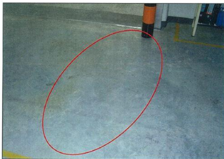
Floor crack at guard pole line G/6 . ( point 2 )
