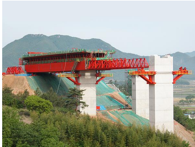
Figure 2.2 Movable Scaffold System (MSS)
