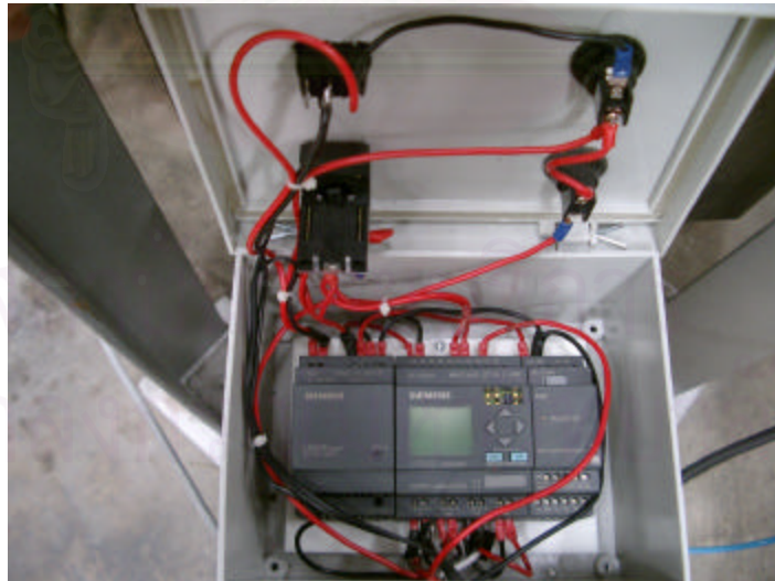
Figure 4.14 Programmable Logic Controller (PLC)
