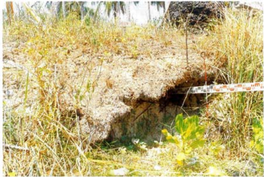
Figure 2.43 Shoreline erosion of about 0.80 meters along Ko Kwang beach
