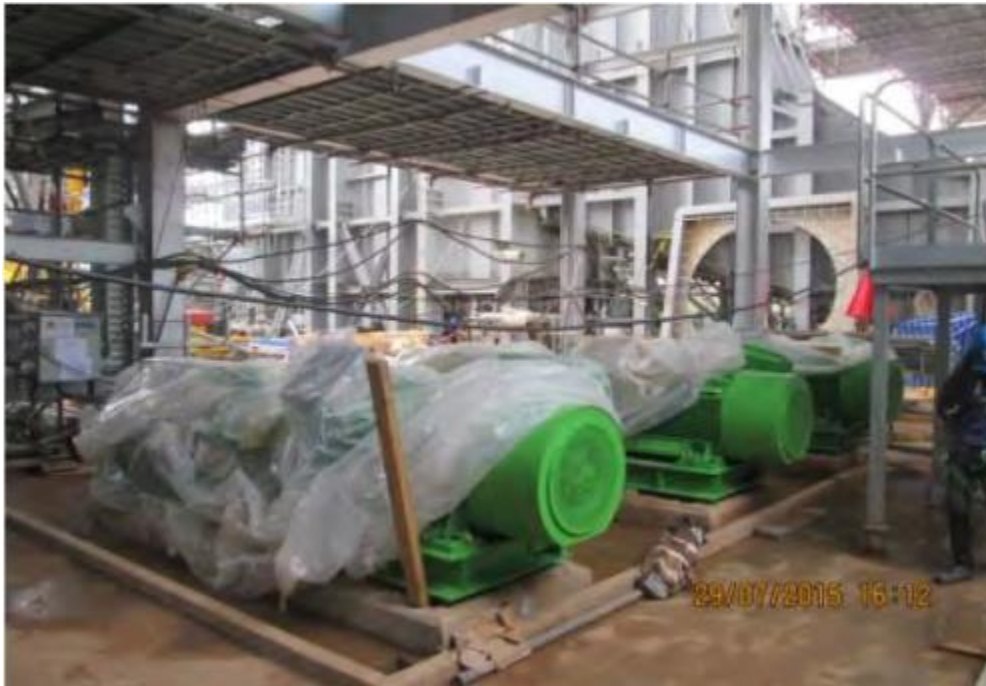
Figure 34 Boiler feedwater pumps installation (Project C monthly reports)
