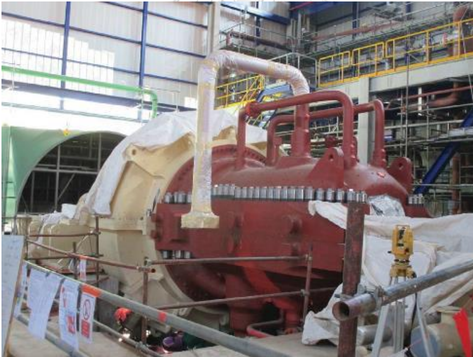
Figure 31 Steam turbine installation (Project D monthly reports)
