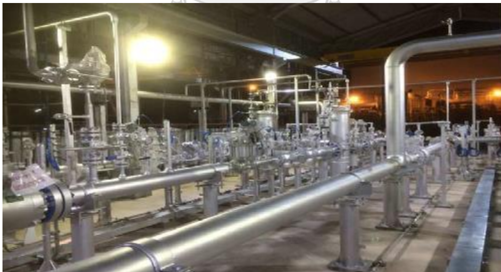
Figure 48 Gas metering installation (Project B monthly reports)
