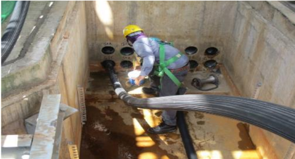
Figure 43 High voltage cable installation (Project B monthly reports)
