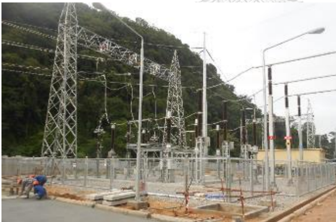
Figure 37 Switchyard installation (Project D monthly reports)
