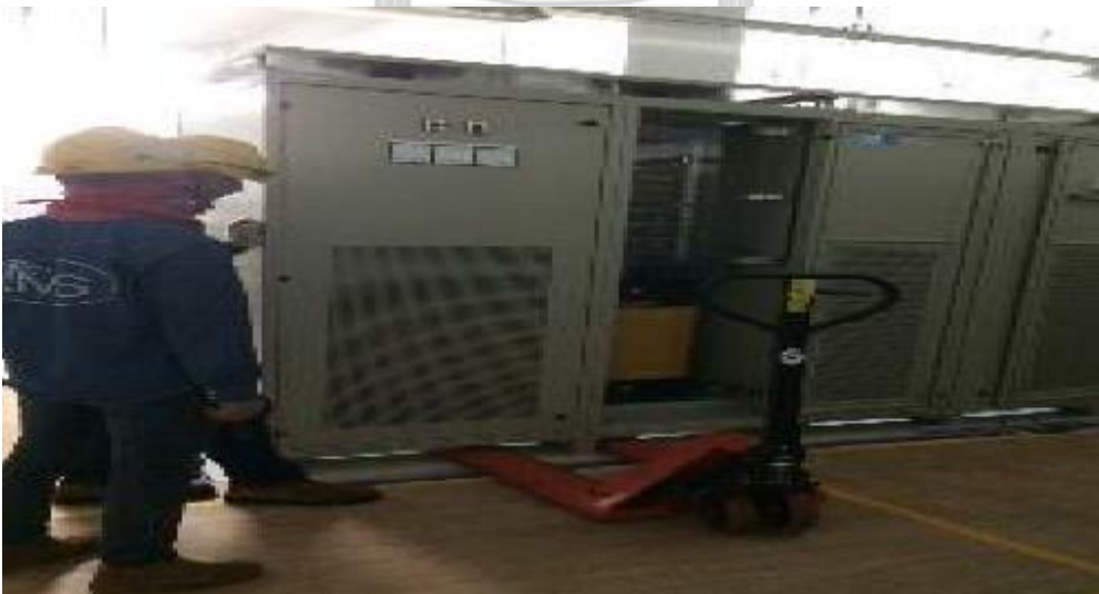
Figure 44 Battery and charger installation as part of the UPS (Project B monthly reports)
