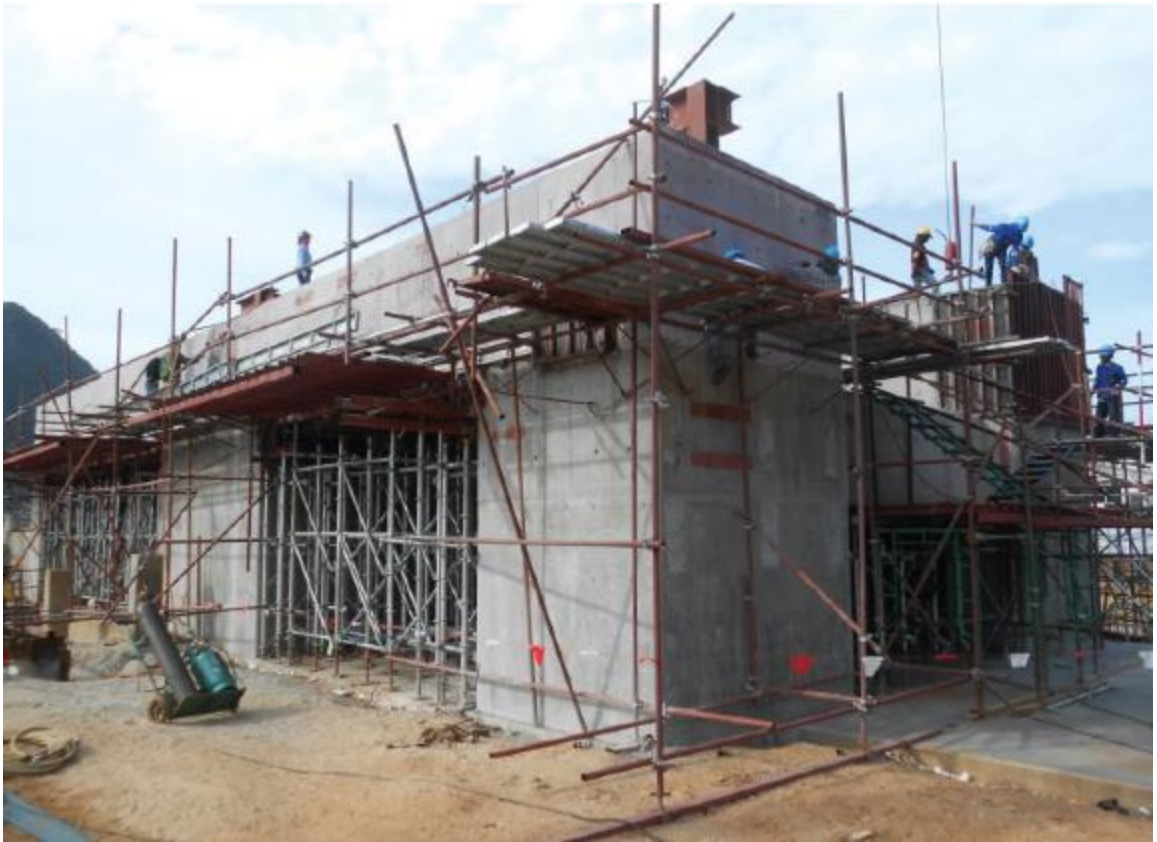
Figure 19 Gas turbine foundation formworks removal after concrete pouring (Project D monthly reports)
