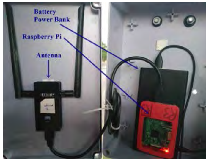
Figure 6.3: Installation of wireless mesh node inside waterproof box over crossover bridge on Phaya Thai Road.
