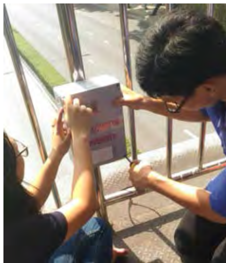
Figure 6.2: Installation of waterproof box at fence of crossover bridge on Phaya Thai Road.
