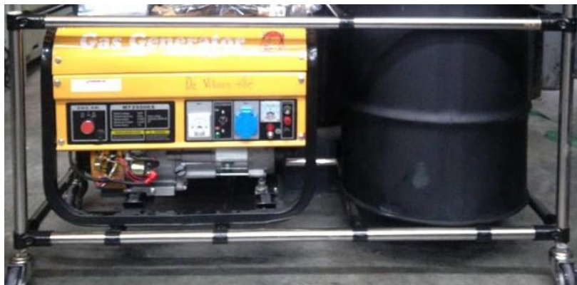
Figure 3.14 gas engine/generator system
