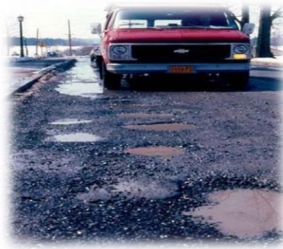
Figure 2.13 Potholes caused by poor drainage [32].
