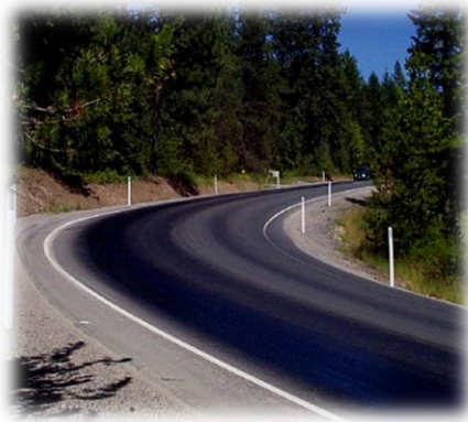
Figure 2.15 Bleeding of asphalt surface [33].
