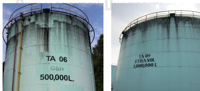
Figure 1.1 Fungal strains on the top wall of an ethanol and gasohol tanks of the PTT Public Company Limited.
