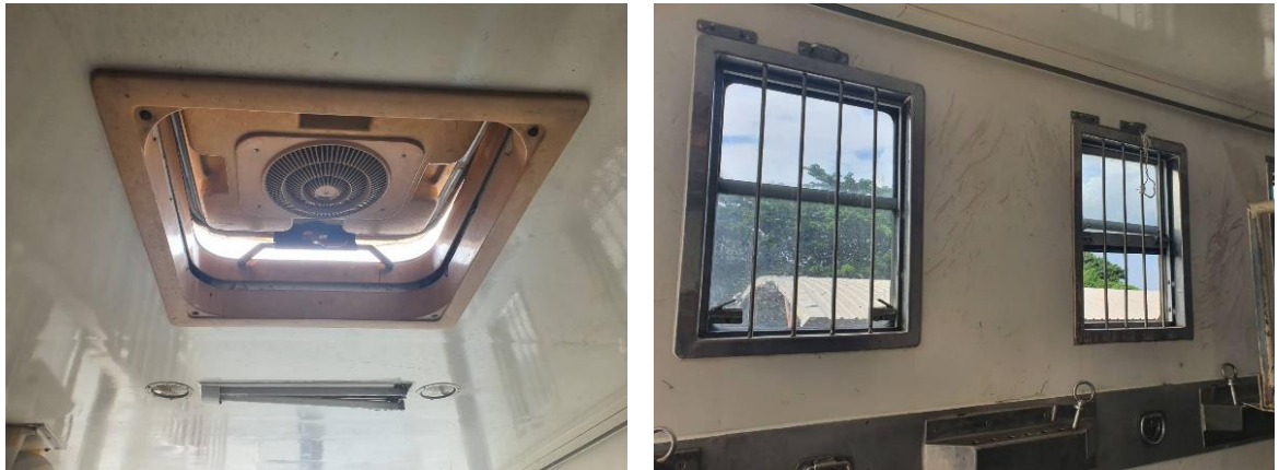
Figure 8: The ventilation system on the roof of the truck and windows inside the air Conditioning truck.
