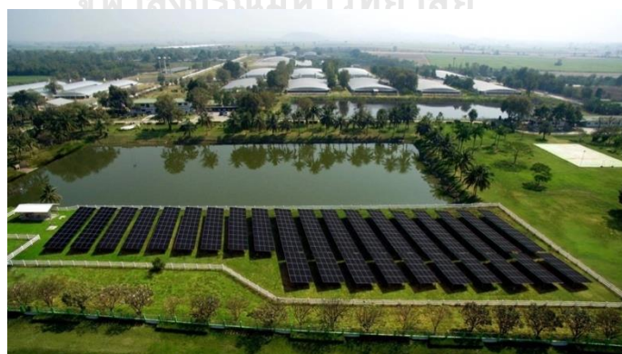
Figure 9: CP's solar panel
