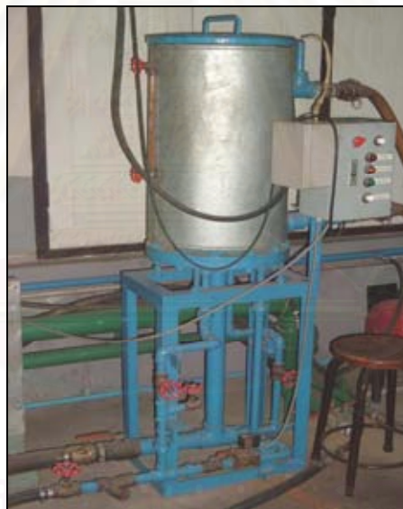
Figure C-4 Cooling water tank
