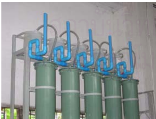
(b) Rainfall pipe and Gas draining pipe
