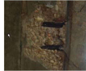
Corrosion at bottom slab, CB7
