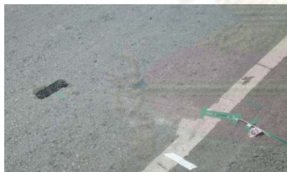
Concrete strain gauges embed on road surface, CB7
