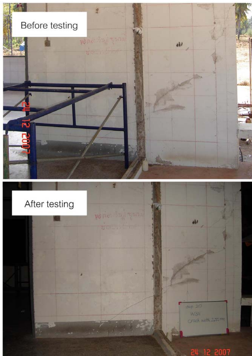
Figure 5-7. Major brick wall with cracks before and after testing
