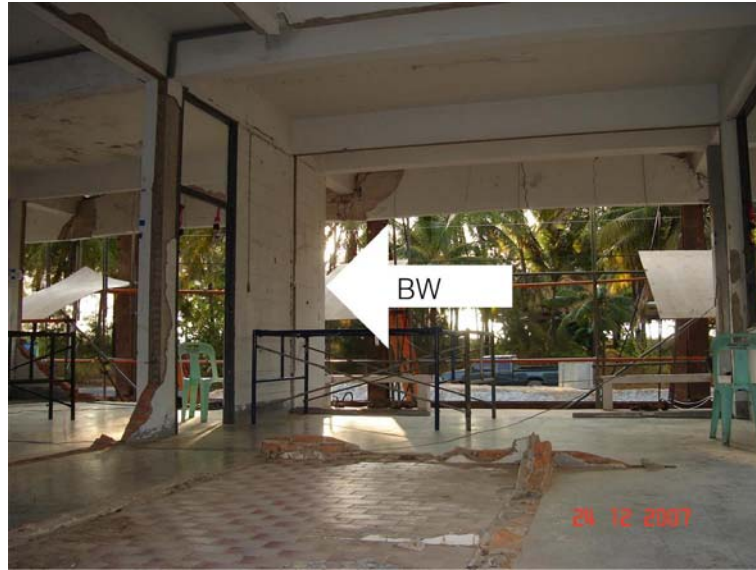
Figure 5-3. The inside view of the building shows the remaining structure and major brick wall (BW)
