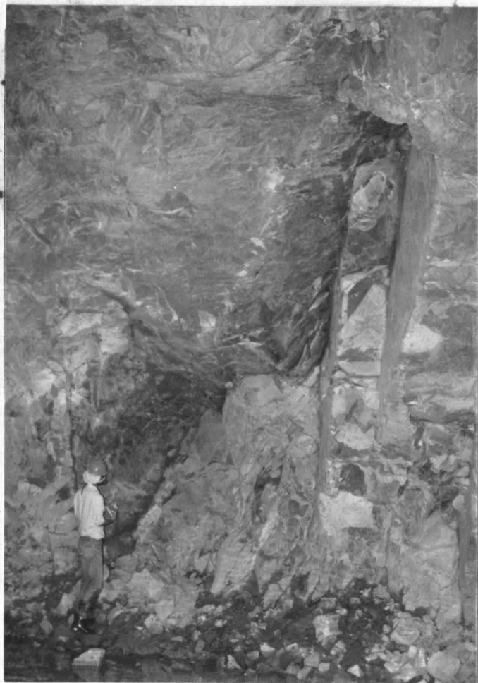
Figure 2.4 Geological overbreak on left wall at cha. 65.00 - 69.00 m in the diversion tunnel.
