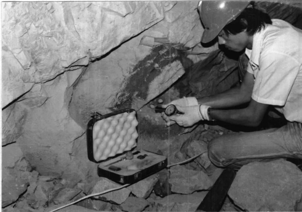
Figure 7.15 Dial gage mounted on the borehole extensometer in pebbly graywackes of diversion tunnel
