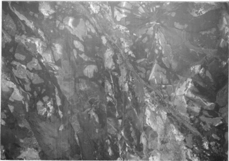
Figure 7.10 Close up of joint conditions on the left wall between the extensometer Section no. 1 and no. 2.
