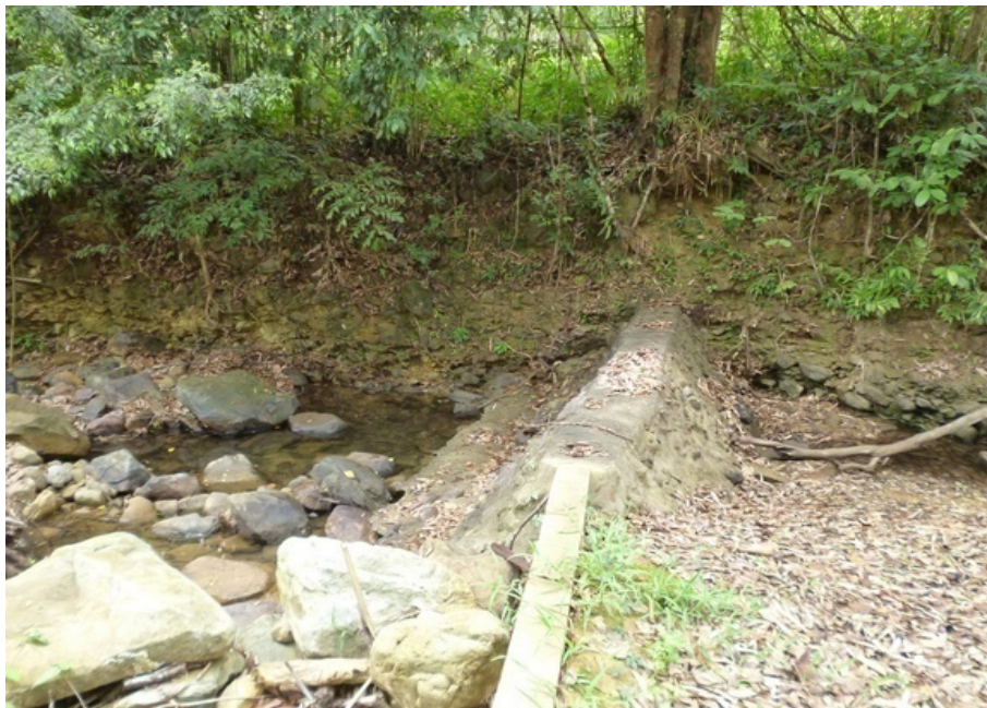
Figure 4.40 The damage of weir after consecutive heavy rainfall.
