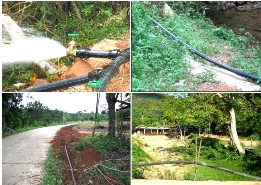
Figure 4.42 The polyethylene water pipelines.
