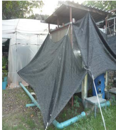
Blower and cooling pad box
