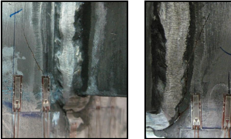
B. Crack occurs from the web-toe.
