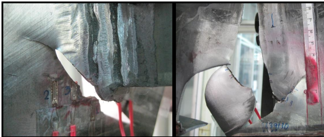
B. Crack on front and back side of girder at failure.
