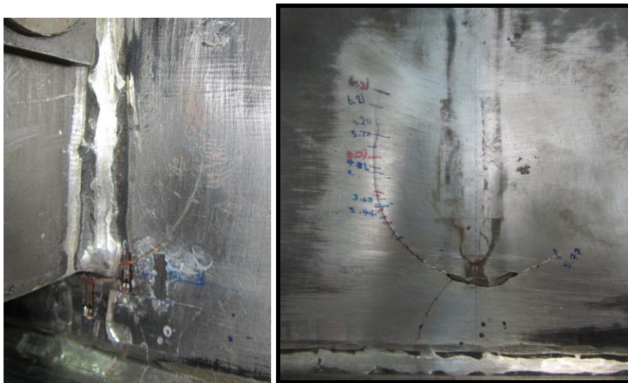
B. Crack on front and back of the girder.
