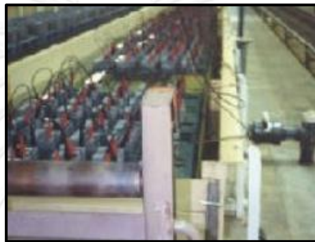
Figure 2-9 Batteries being charged by wet charging [19]
