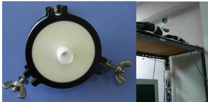
Figure 3. 4 Particle filter connected with outdoor installed tube line.
