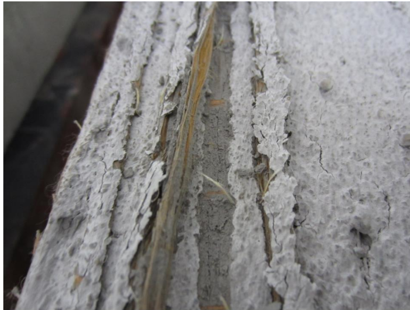
Figure 4. 2 Thin layer of cementitious after debonding
