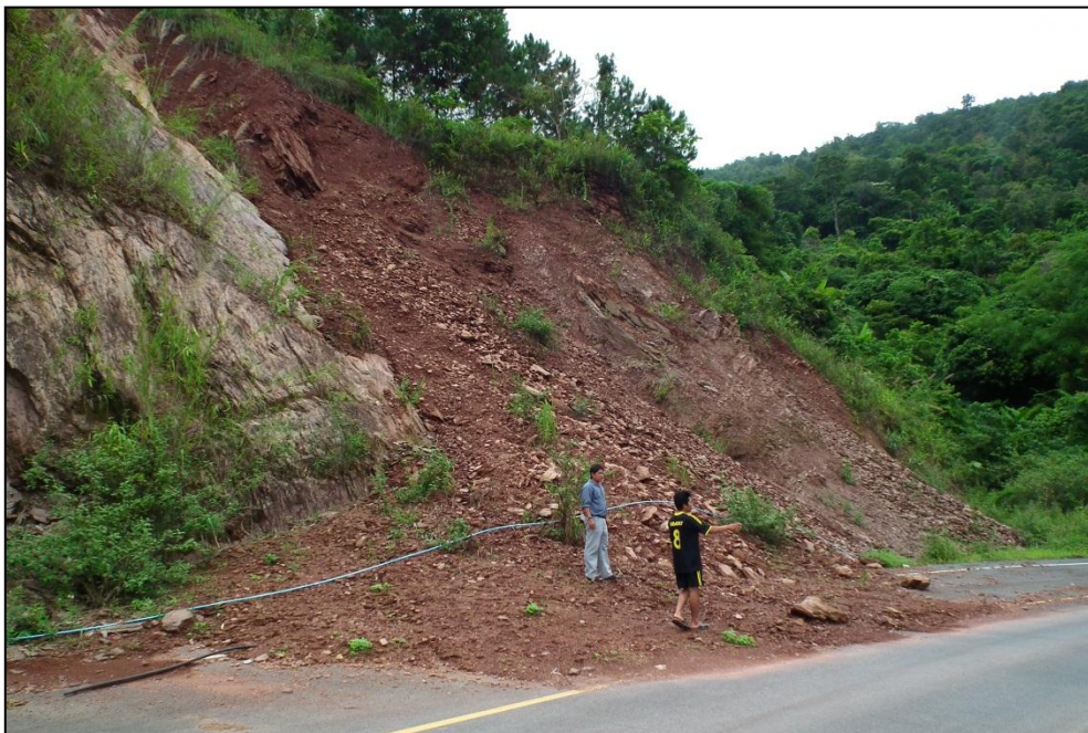
Figure 1.3. Landslide occurrence (cut slope failure) in the Ban Nong Pla area.
