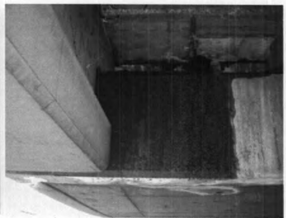
(c) Water leakage
