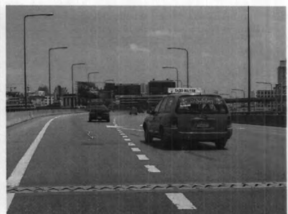
(e) Maintenance cost on expansion joint
