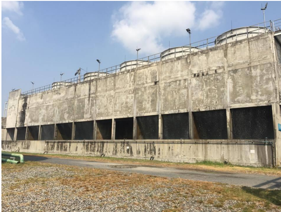
Figure 3.2 One of cooling tower units in co-generation power plant
