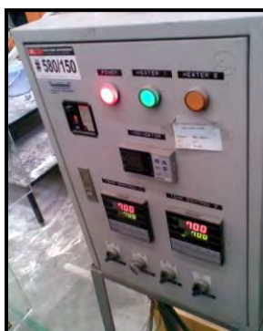
Figure 3.9 Temperature control system
