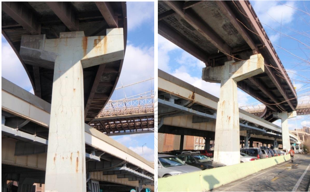
Figure 1 Existing corroded RC bridge located in an aggressive environment (Photograph was taken by Mitsuyoshi Akiyama)
