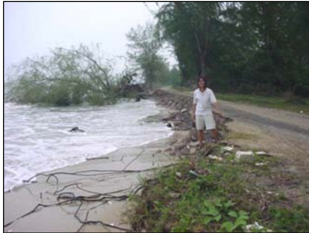
Figure 4.15 Eroded area at Laem Talum Puk UTM 627426 E/ 940764 N shows road in the area had eroded
