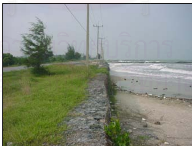
Figure 4.14 Rubble-mound Revetment at Ban Kho Fai, Ka Nap Nak sub-district, UTM 642216E/906809N
