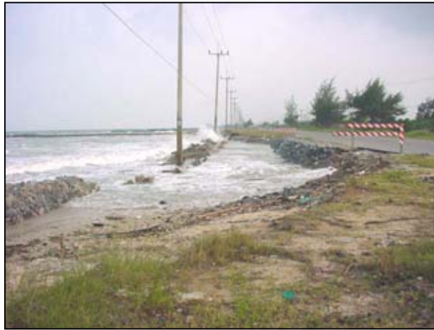
Figure 4.21 Pak Phanang-Song Khra road Km. 19-20 in Ban Kho Fai, Kha Nab Nak sub-district UTM 641826 E/ 908579 N shows the violence of wave that insist to the road
