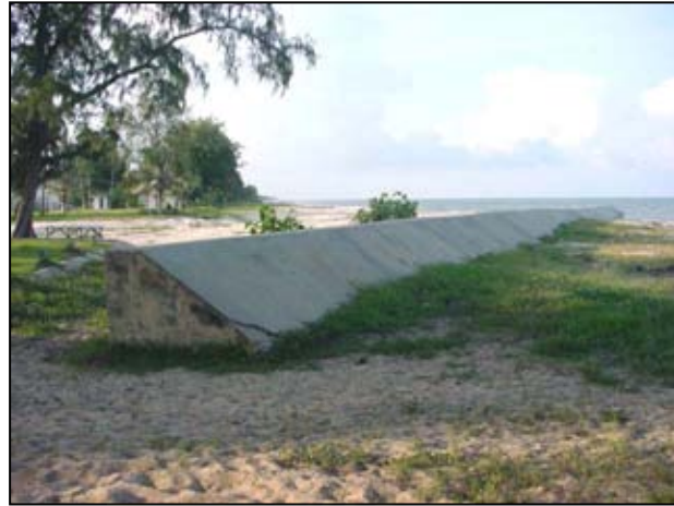
Figure 4.12 Jetty at Pak Ra Wa canal, Ban Na Thod, Na Saton sub-district, UTM 647666E/876661N
