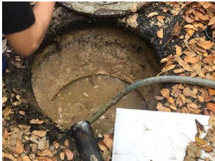
Figure 3.1 septic tank at Chulachakrabonse Building
