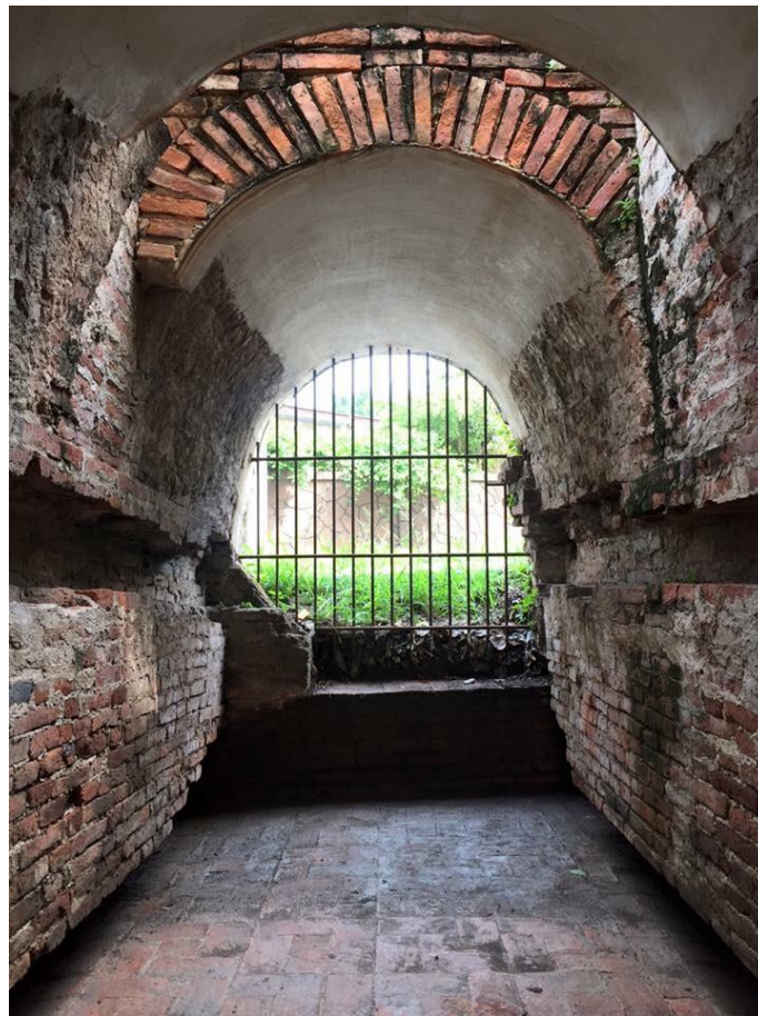
Figure 5.30 Water tunnel within the city moat seen at Pratu Khao Puerg Fort
