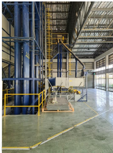
Figure 9: Image of Dry Mill
