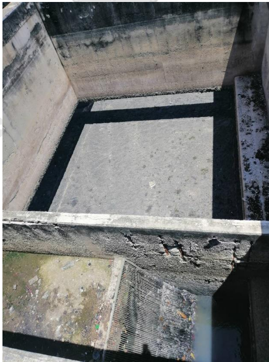
Figure D2 Influent and grit chamber
