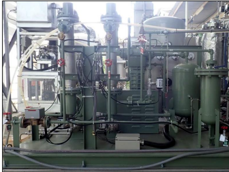
Figure 42 The first gas compression unit
