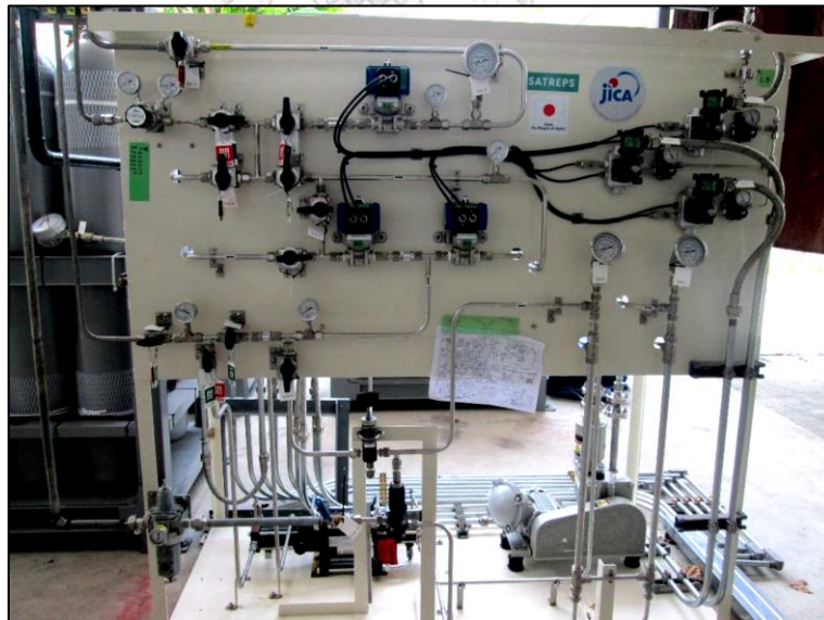
Figure 43 The second gas compression unit
