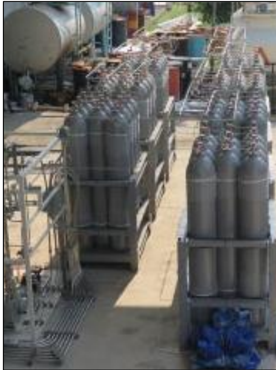
Figure 44 Gas storage tanks (Buffer Tank)
