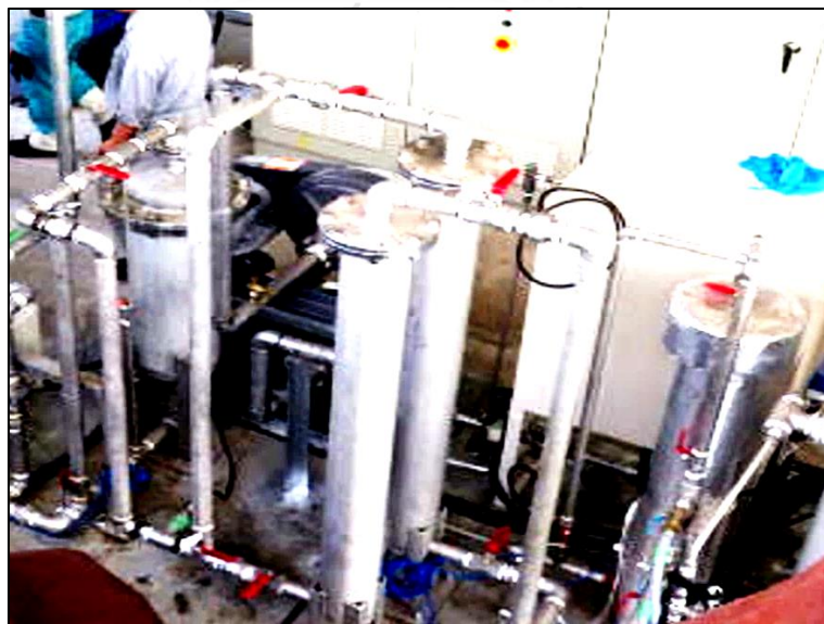
Figure 40 Set of Gas cleaning Unit a) Mist separator, b) Desulfurization, c) O 2 remover
