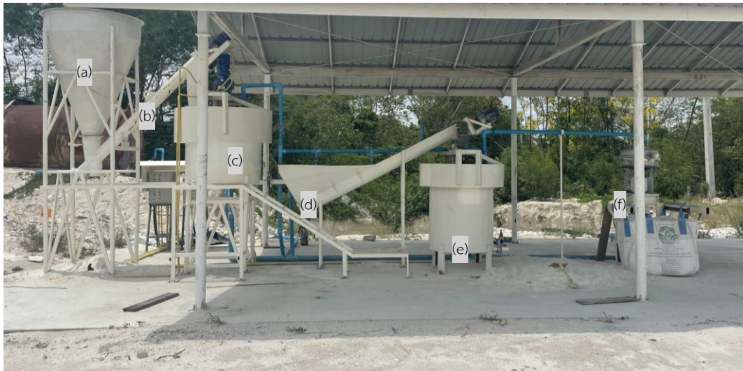
Figure 3.4 Equipment used for pilot experiments: (a) hopper, (b) screw feeder, (c) attrition scrubber, (d) spiral classifier, (e) impelled clarifier, and (f) rounded screen.
