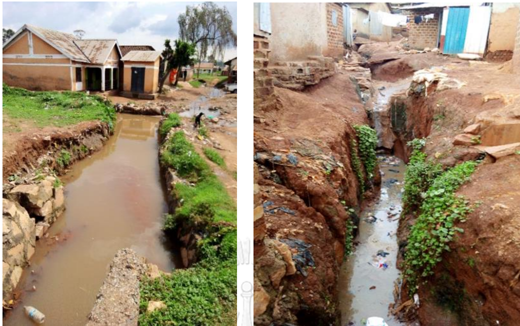
Figure 6: Blocked drainages in Kanyanya and Banda Slums.
