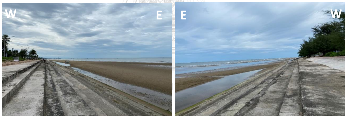
Figure 32. Pictures of the coast at Station 3, a stepped seawall covered the coast made by the government.
