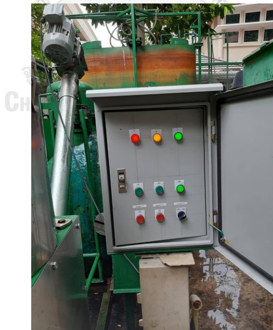
Figure 16 Controller unit of the food waste treatment system
