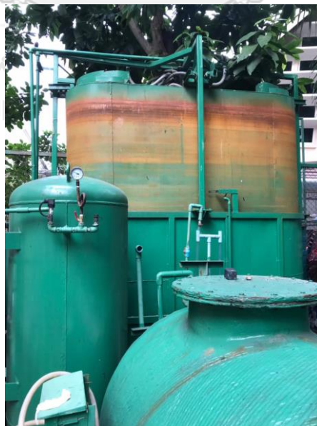
Figure 23 Biogas holding tank and compressed pressure tank
