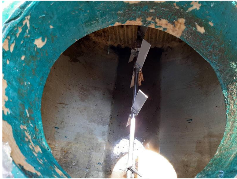
Figure 17 Digester unit (inside)
